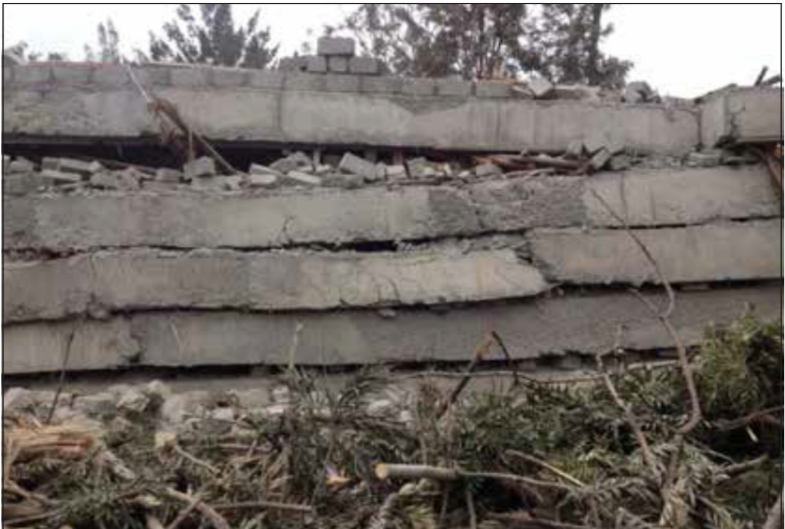
Figure 6.3: Collapse of a building under construction at Laiser Hill area Ongata Rongai Town, Kajiado County in September, 2015
